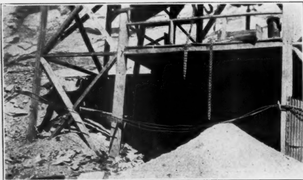
Loading Platform to Roll Crusher
